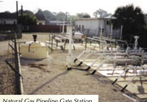
Natural Gas Pipeline Gate Station in Titusville.
